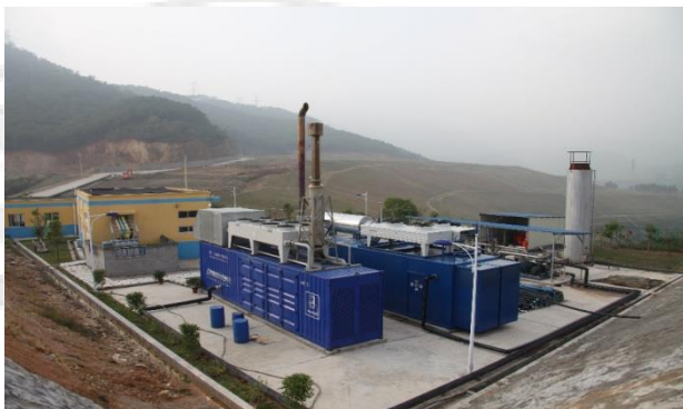
Landfill gas treatment
